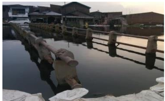
Fig. 7 Situation of a sinking bridge in Jakarta, Indonesia [3]
