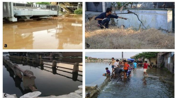
Fig. 1 Sea inundation (a), cracking on the buildings (b), sinking on the bridges (c) and dikes (d) due to land subsidence occurred in Semarang and Jakarta, Indonesia [3]
