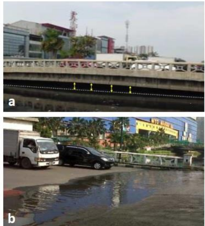
Fig. 6 Situation of two sinking bridges in Semarang, Indonesia [3]
