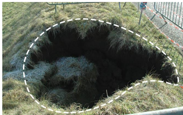
Fig. 11 Sinkhole at the top of a Loire River dyke. Adapted from [35]
