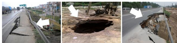
Fig. 10 Sinkhole Collapses on the project. Adapted from [30]
