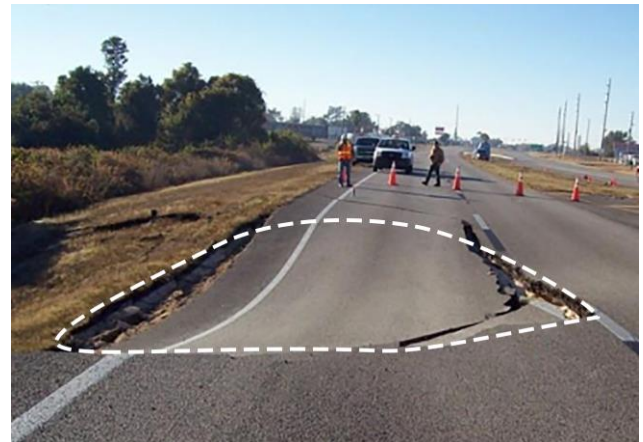
Fig. 7 Cover-Subsidence Sinkhole; formed underneath a US27 in Polk County, United States of America. Adapted from [4]
