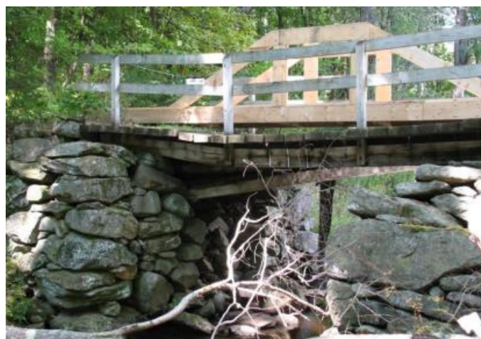
Fig. 12 Sinkhole of Sackett Harbor's Bridge. Adapted from [39]
